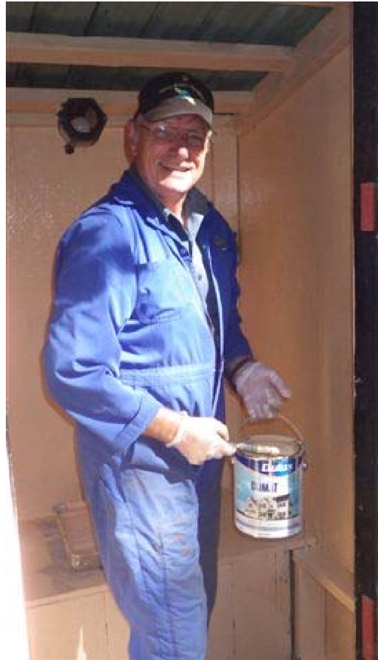
John to scrape and repaint biffy 1, the fire damaged one
