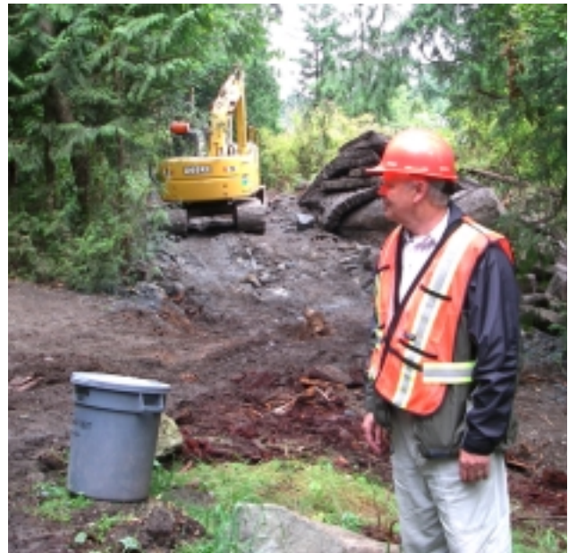
Jim McCoy keeps a watchfull eye out for pedestrians and vehicles while the excavator cleans out the rock which had just been blasted loose in the channel.
