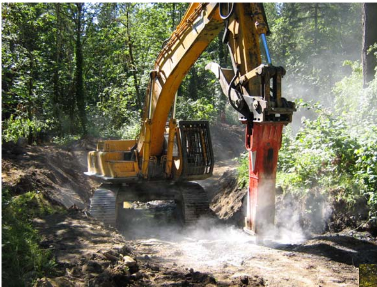
An excavator with a jackhammer attachment formed the channel into the bedrock.
